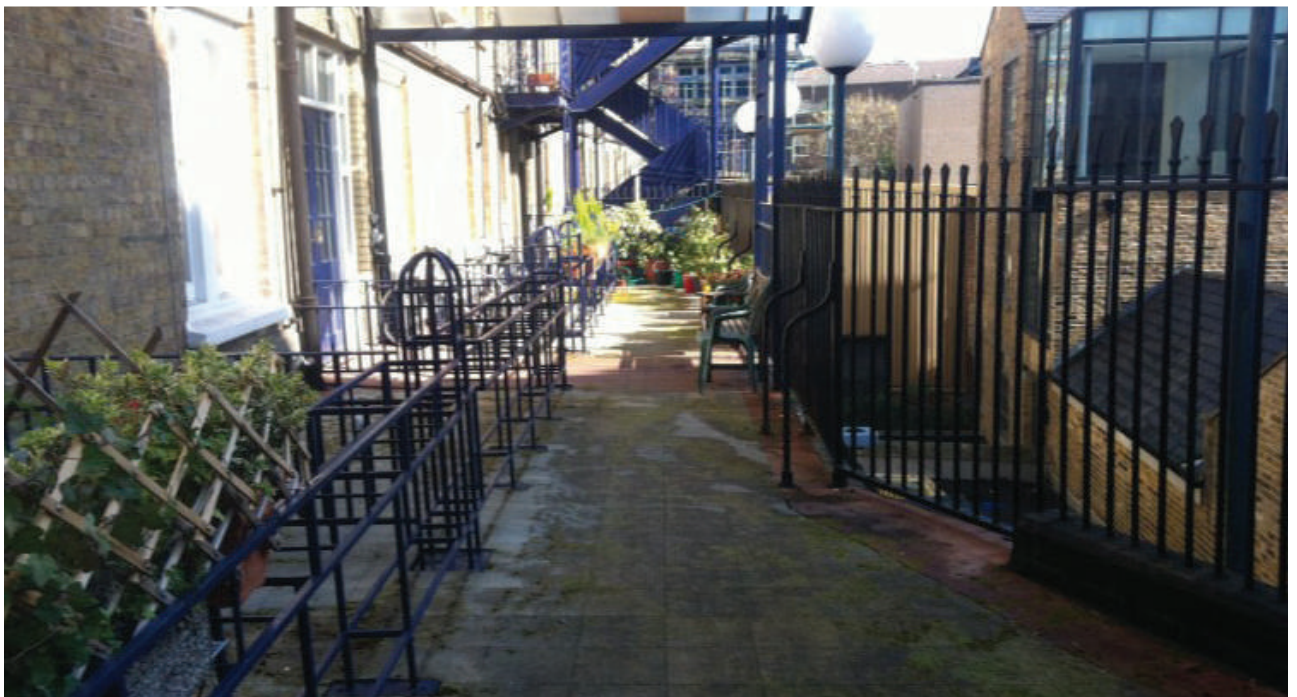
Rosebery Square East Residential Flats, Clerkenwell, London Size 900m 2 IKO Polimar FCS Walkway System was installed to replace the failing material on top of the mastic asphalt substrate. Because IKO Polimar FCS is fast-curing, it has enabled traffic by the residents to be acceptable within minutes of being applied. Contractor: Capital Roofing System: Cold Applied Liquid
