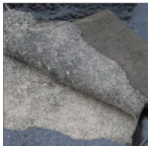
Failed peel - easily pulled from the substrate
