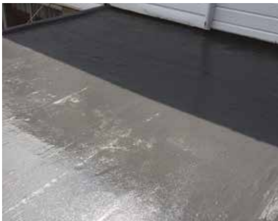
Apply a further coat ensuring the total minimum coverage of 1.2L/m 2 is achieved to finish the roof
