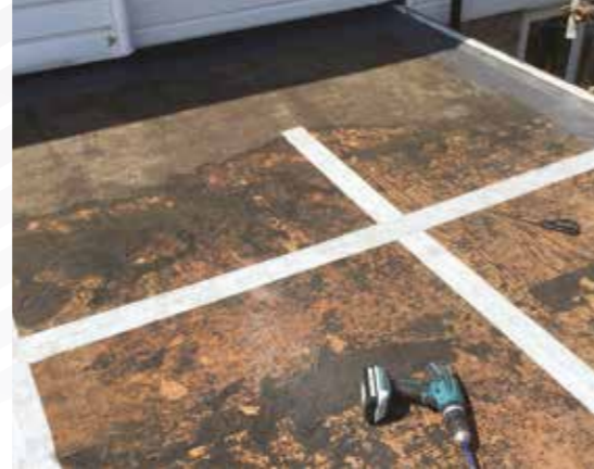
Once the surface has been cleaned and primed use FIX-R Jointing Tape to cover joints in the surface
